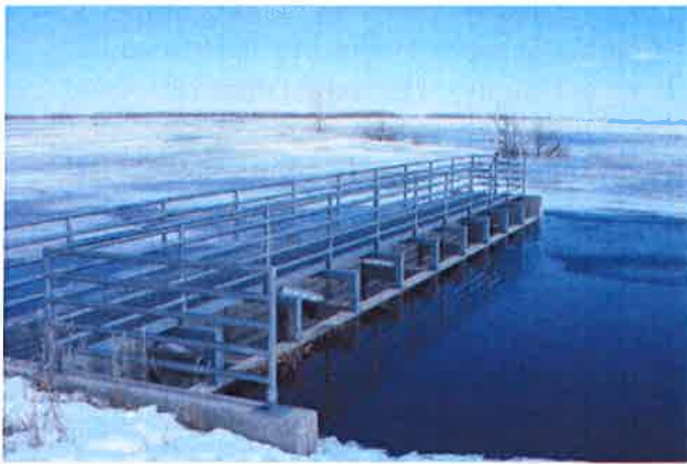
Outlet Structure at Ross #7 Impoundment
